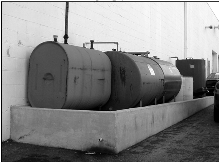
Figure P.6 Secondary Containment of Storage Drums Behind a Car Repair Shop.
