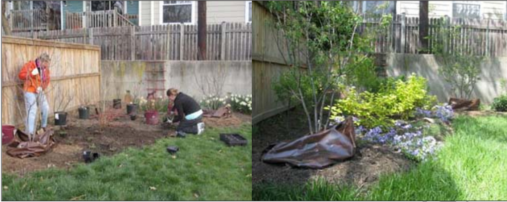
Figure 3.12 Demonstration sites exist throughout the District to promote downspout disconnection, removing impervious pavement, and promoting native plants.
