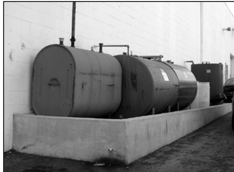
Figure 2: Secondary Containment of Storage Drums Behind a Car Repair Shop
